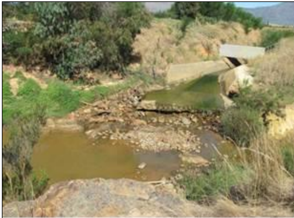
Figure 20: Highly eroded discharge point (photo courtesy Nemai Consulting)
